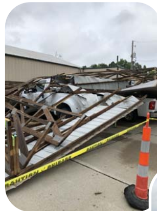
Wind damage at the O'Fallon Project site. For- tunately only minor dam- age at the Rain Garden. MN Elaine Browning
